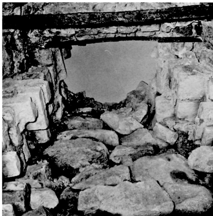
34 2E1?. View of the east fireplace in the casemate showing the top of firebox and metal braces. Camera facing up. No scale (2E-3154 X).
